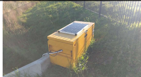
Autosampler with solar panel setup at the inlet of Sorrento Way SQID
