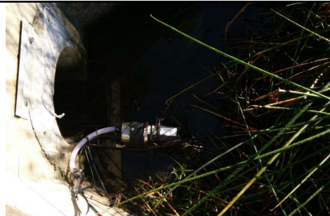
Pump with plumbing to autosampler, flow meter and depth sensor install in the low flow outlet pipe
